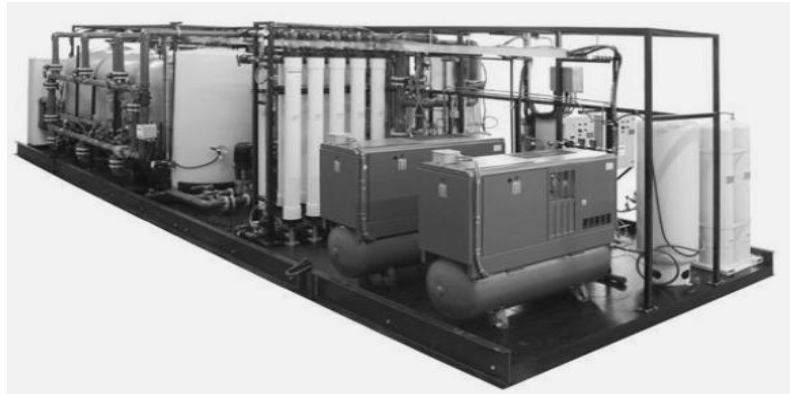
Figure 2 A modular unit of the Dagua water treatment plant
